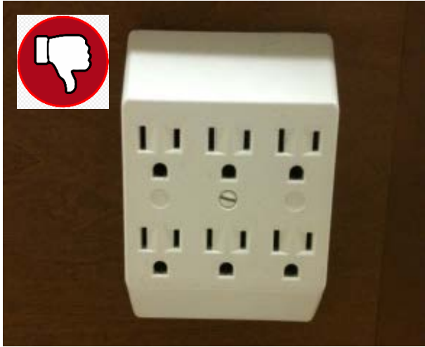
A prohibited multi-outlet adapter (no circuit breaker).
