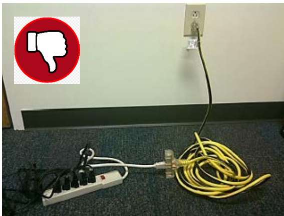
Improper power strip use; plugged into extension cord. Power strips must be plugged directly into an outlet and extension cords are for short term use only.
