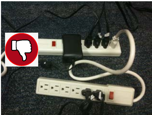
Power strips may not be "daisy chained."
